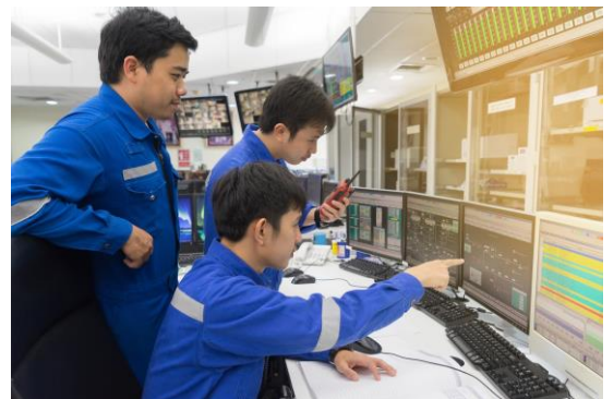
Experion HS is a powerful software platform built on the proven technologies of the Experion PKS platform and provides an integrated, reliable and secure environment with ControlEdge HC900.
